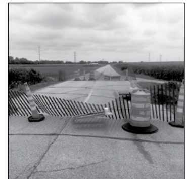
July floods brought closed roads and more Pike River bank erosion. We brought the U.S. Army Corps of Engineers in August.
